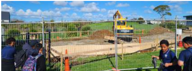
Thanks to these guys for the early finish last Friday (burst water pipe) - just kidding 🤡 Poetiara's new building will look mean once it is all done!
